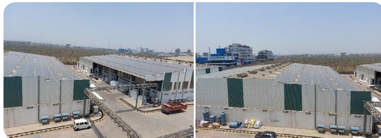
Solar Panels installed in Warehouse of Dahej plant which leads to reduced green house effects
